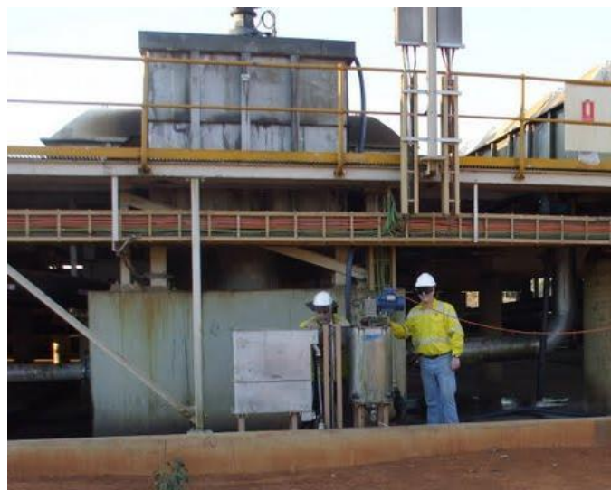
Figure11: Turbulent Technologies Pilot Facility Lady Annie (LA) Copper Mine, Australia
